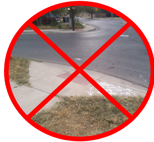
Diagonal Curb Ramps No Longer Desired
