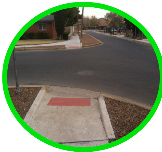
ADA Compliant Directional Curb Ramps
