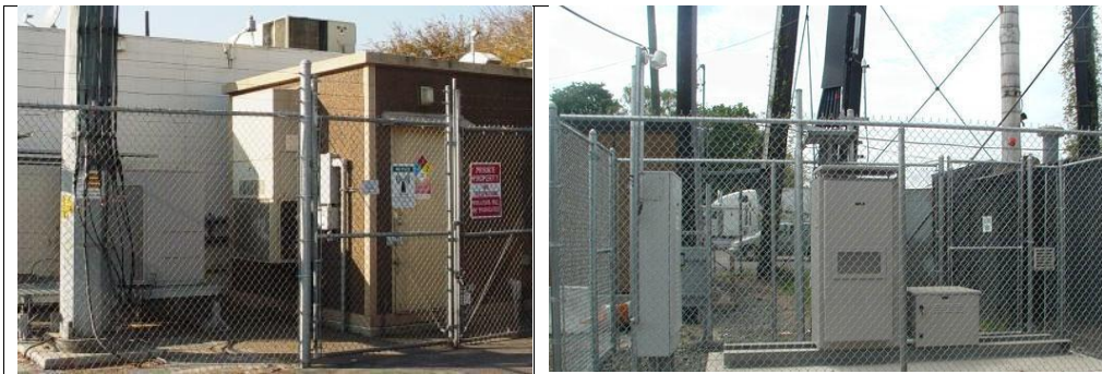
The ground equipment is not screened with a rockwall or wrought-iron fence and no additional landscaping is provided to screen the equipment.
