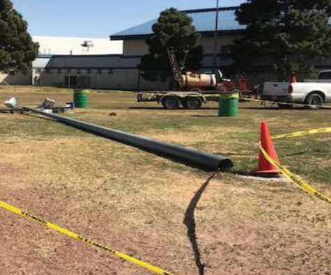
Boa Park Ballfield Light in wind event due to at base
