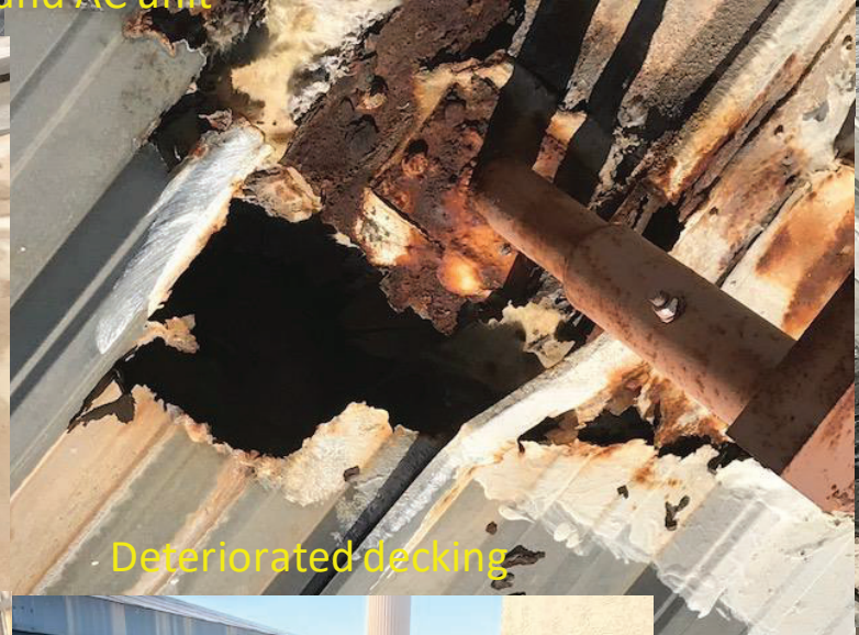
8600 Montana - Deteriorated decking and AC unit
