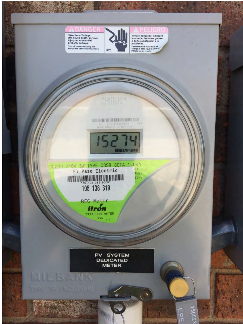
Solar PV Dedicated Meter or REC Meter
